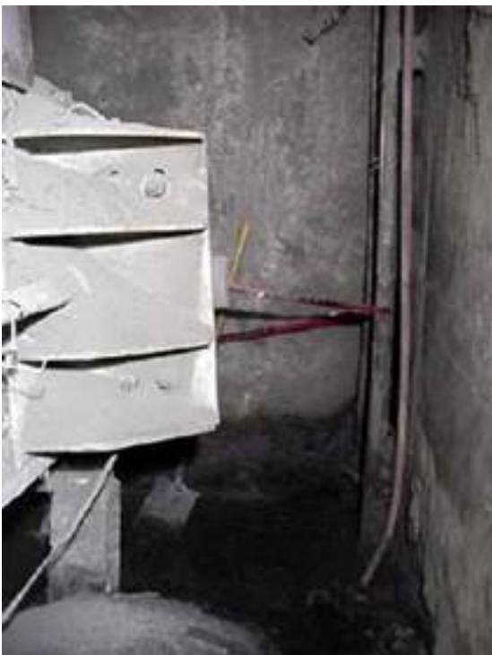
Fatal accident site
